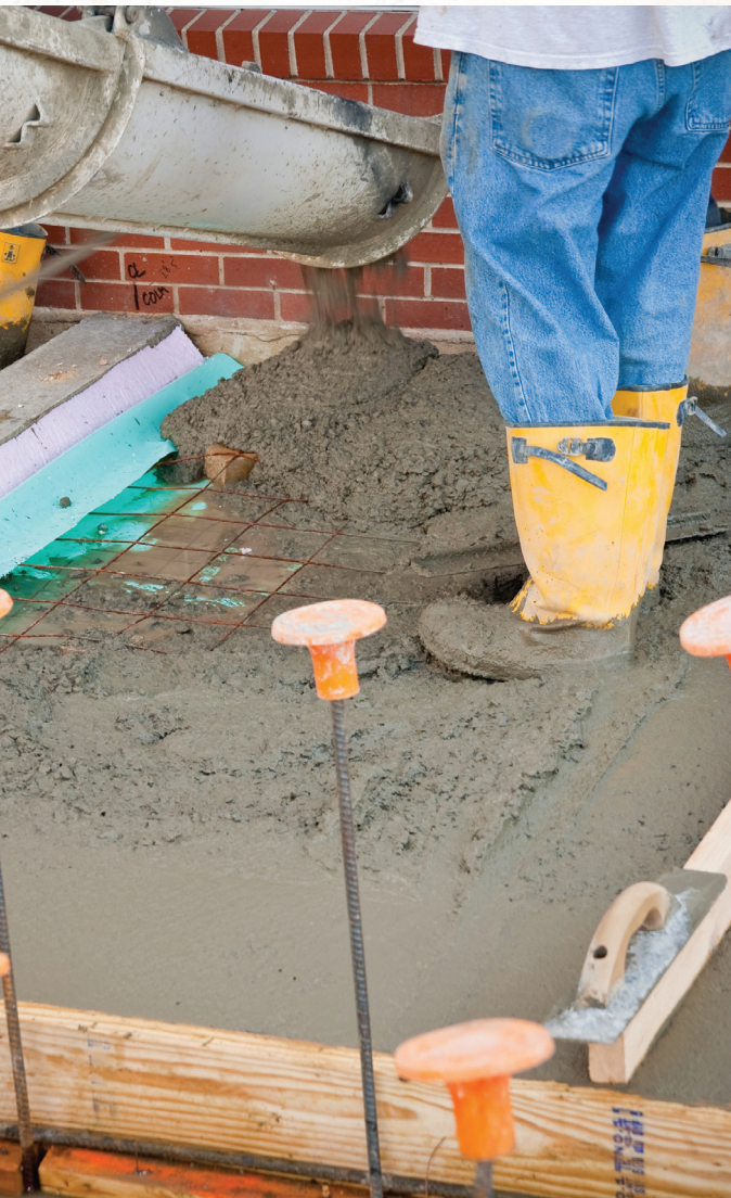
Sections of concrete shrink to leave a gap of anything up to 25mm wide between slabs
